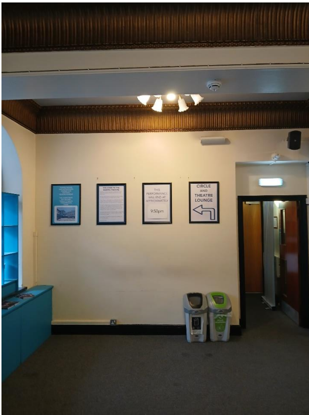
This image shows where the cables for the CCTV will have to run for the new management office.
