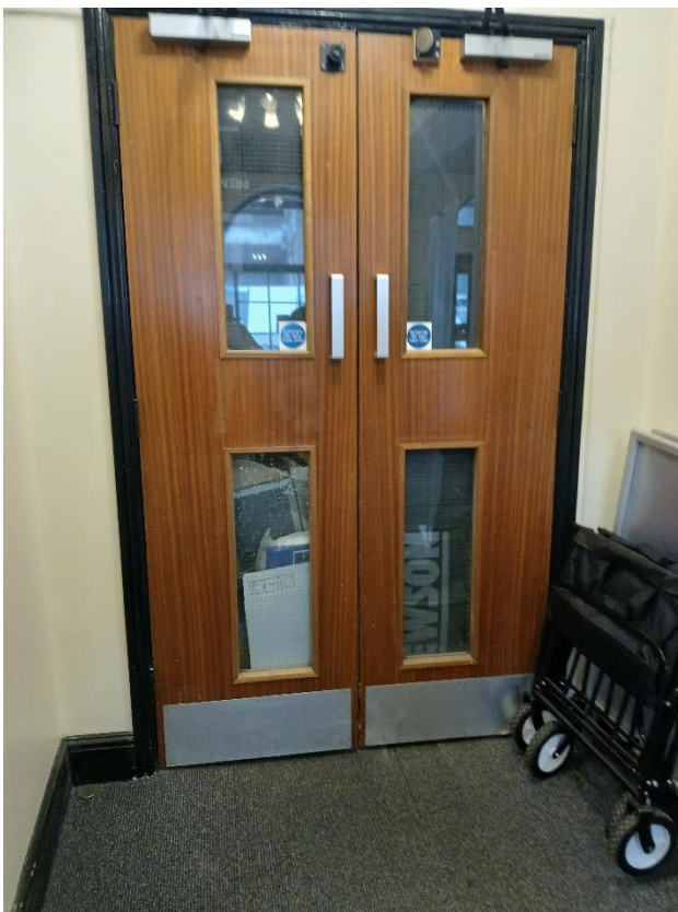
This image shows blocked off doors to allow hoardings to be erected as shown on the floor plan.
